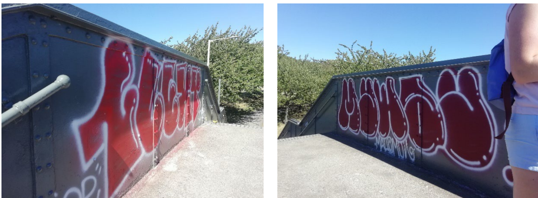
Figure 15: Graffiti on the existing bridge is an issue
