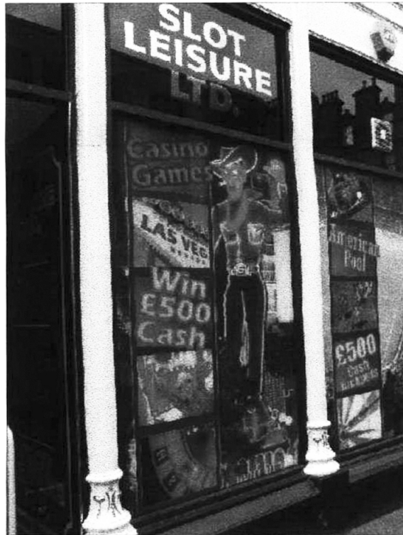
THIS WINDOW TO BE REMOVED SIGN OVER TO BE RETAIN & ALTERED AS REQUIRED
