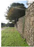
Mature sycamore undermining stone wall Possible requirement for Engineers report & repointing with lime
