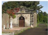
Former stable, stone, roof in disrepair Potential to be used if re-instated
