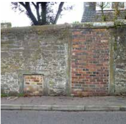
Insensitive repair work
