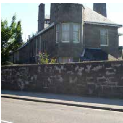
inappropriate repairs to boundary wall
