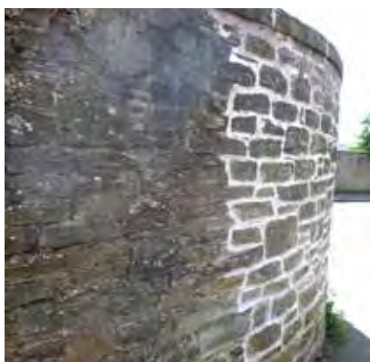
Insensitive wall repairs
