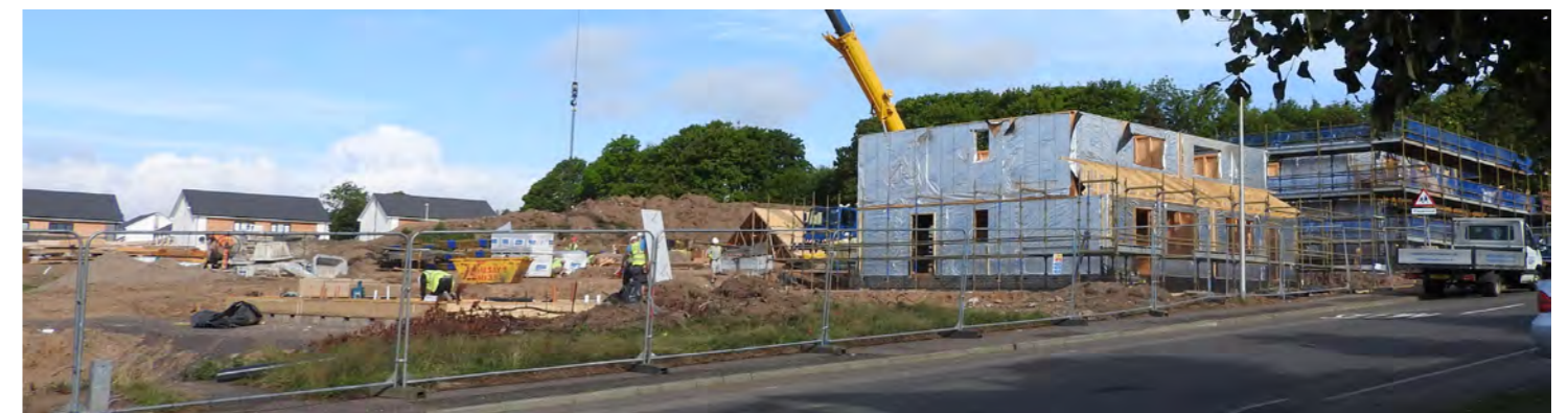
Figure 13: Examples of new developments delivered or under construction within Whitfield including Salton Crescent, Summerfield Avenue and Whitfield Loan.
